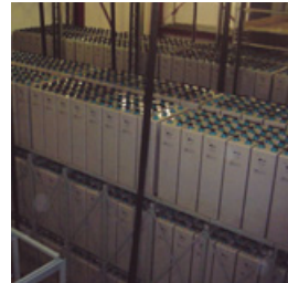
Colt Telecom in Amsterdam 24 OPzV 3000
