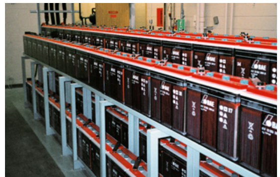
UPS application in USA 6 V 11 OGi 275
